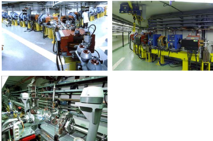
Fig. 28. Particle beam transfer lines (CERN TS-SU library)
